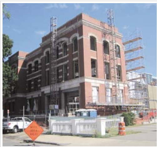
The Springfield Data Center, currently under construction on the former Technical High School site.
